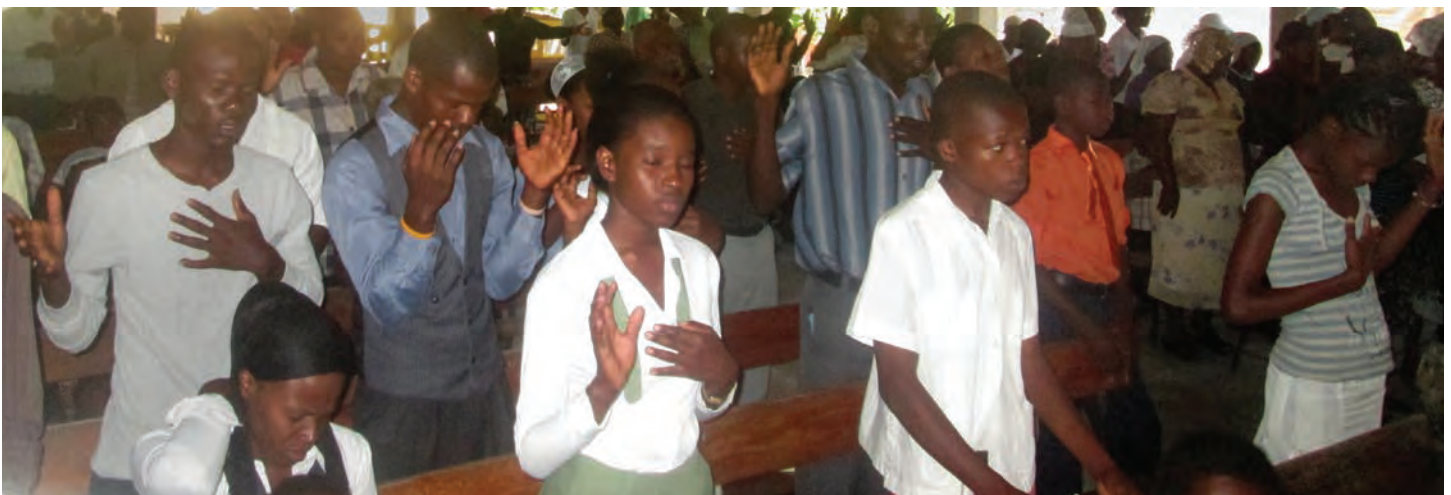
Middle: From roof trusses to church benches, our church construction in Haiti is 100% Haitian built—which leads to greater respect and dignity. Bottom: We rejoice with the people of Brache-Gilles, Haiti, as their new church building is finished and this facility is open to the community throughout the week for other activities.
