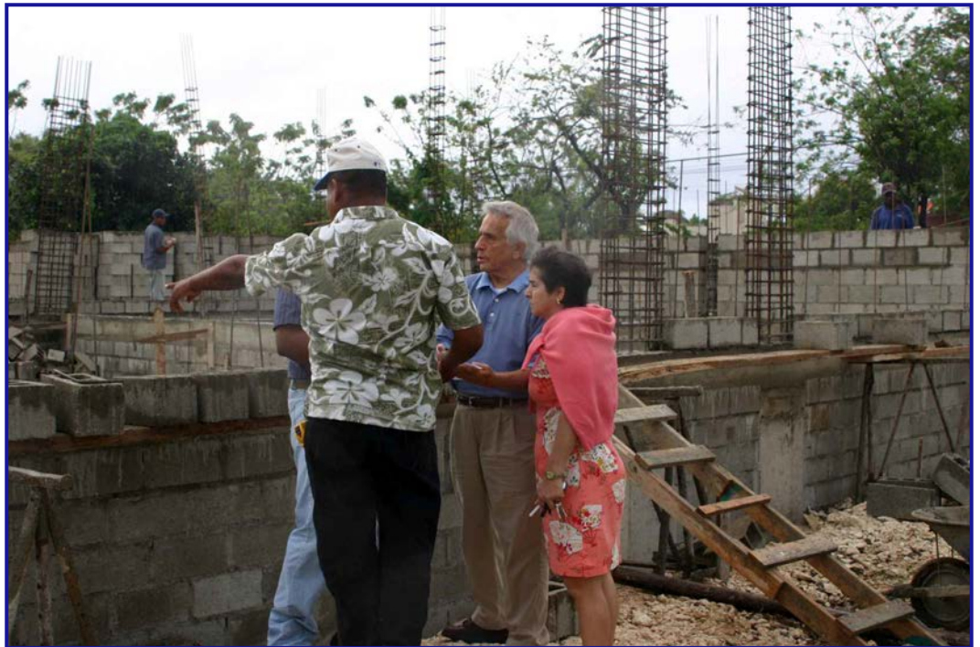
George and Jeanne planning the placement of doors and windows in the clinic.
