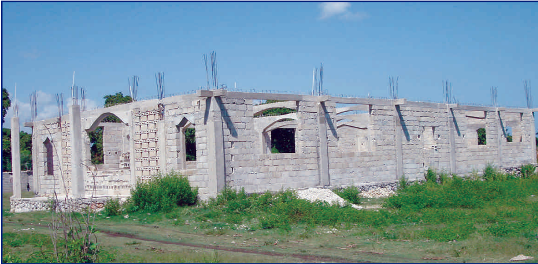
The construction of the Santo Church is on schedule to be completed by the opening of school in September. This church is strategically located across from a voodoo temple.
