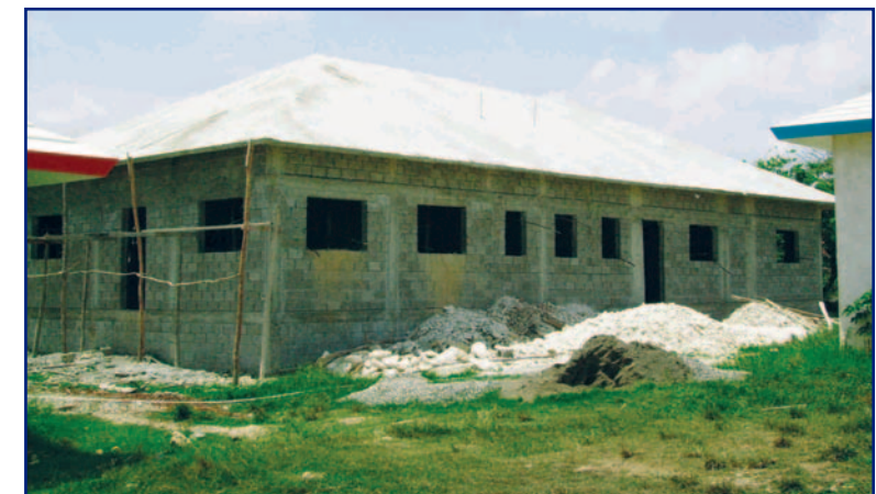
The Community Health Center roof is up and we are on schedule to complete the construction by September.
