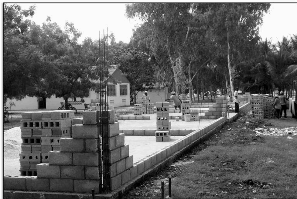
The building is going up thanks to your faithful prayers and support.
