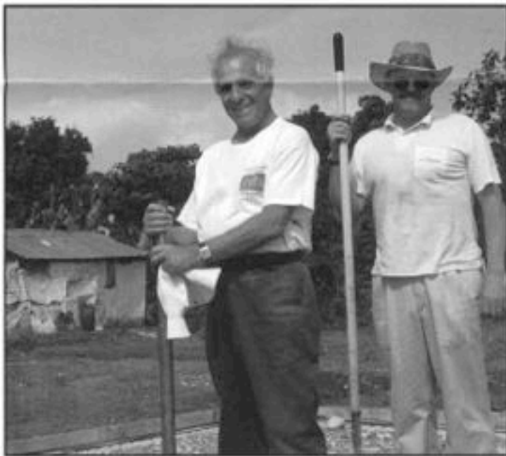
Pastor George working on the widow's house with Dr. Tom Bailey from House on the Rock Church in Pennsylvania.
