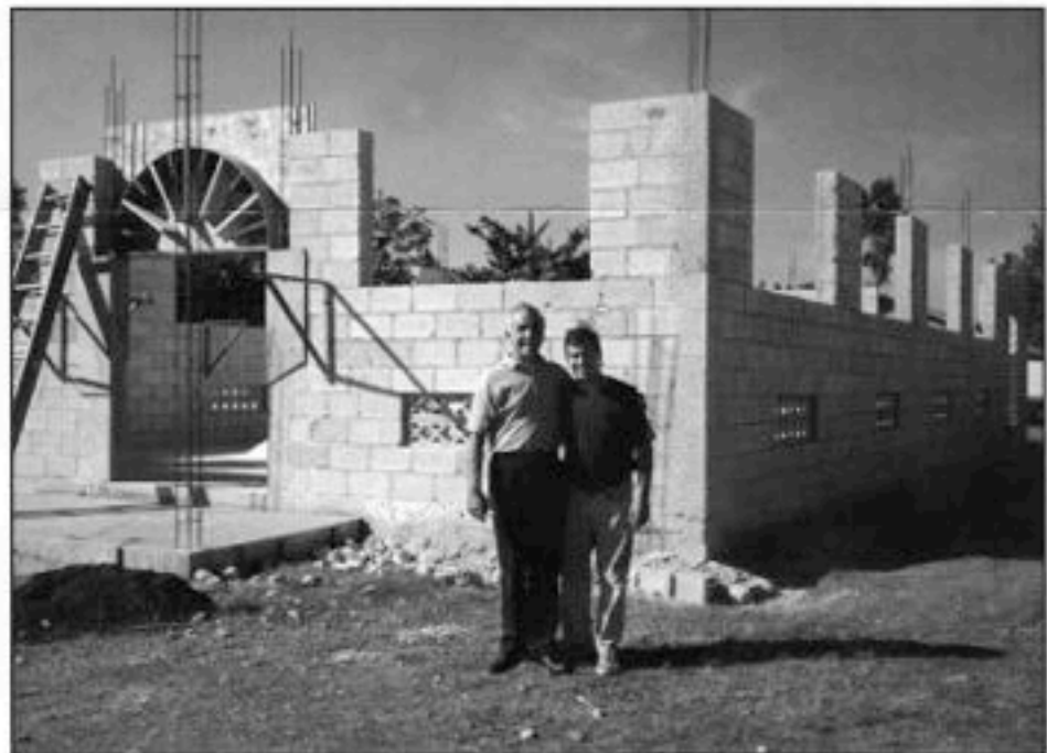
Pastor George DeTellis and son Timothy marvel at the rapid construction of this new church in Masson.
