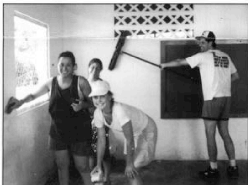
Many of the crusaders painted school classrooms. This classroom at the Bordmer school was being washed in preparation for its painting.
