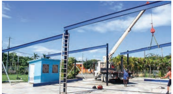
We are thankful that we are able to replace the tent with a metal structure that will last much longer.
